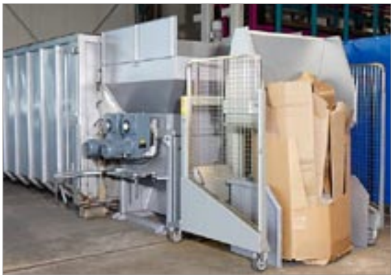
Electro-hydraulic tipping device
